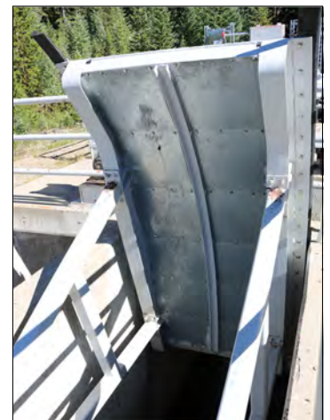
Cunningham Diversion gate.
