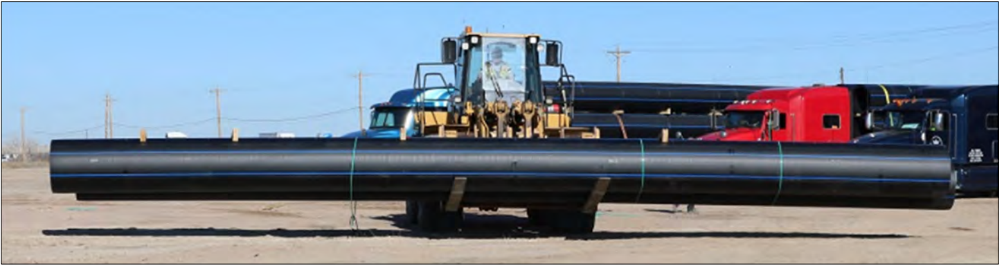
The first load of 30-inch pipeline to be used in building the Trunk Line arrives at the construction mobilization site in March.
